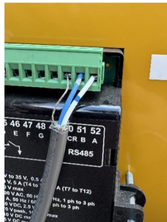
Modbus Connections on Controller
